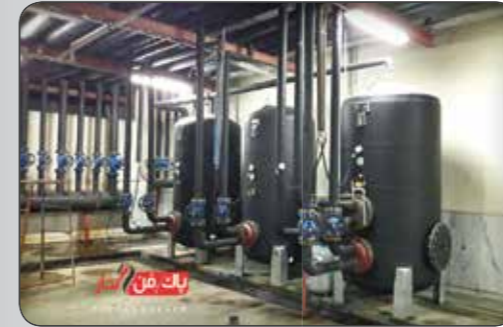
Firebox hot water boiler
