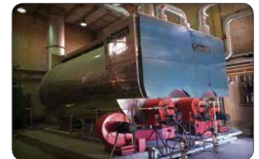
Deaerator, Boiler & Other Boiler Room Accessories Combined Cycle Power Plant Damavand
