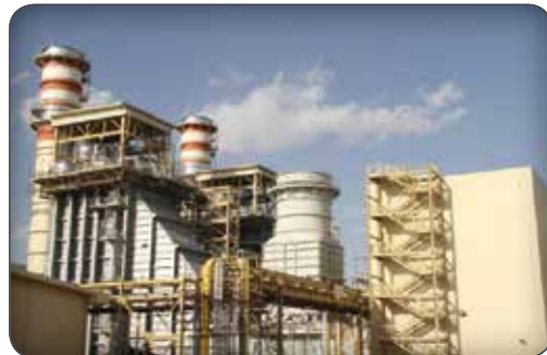
Heat Recovery Steam Generators (HRSG) Yazd Taban Combined Cycle Power Plant
