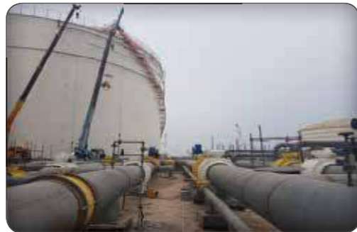
Construction & Installation & Pre-Commissioning of AG /UG Piping & Mechanical Equipment and BOG Unit of AGTP Petrochemical Co.
