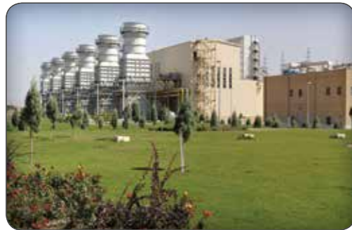
Three Pass Steam Boiler & Other Boiler Room Accessories Parand Combined Cycle Power Plant
