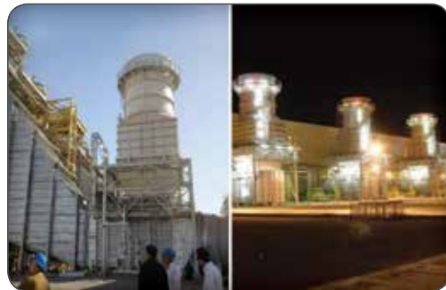
Construction of 160MW Gas Turbine units (SakhteTajhizat Sepahan Company- STS (Mapna Group))
