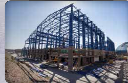
Fabrication and installation of Steel structure of Main shop of Sangan Concentrate Project
