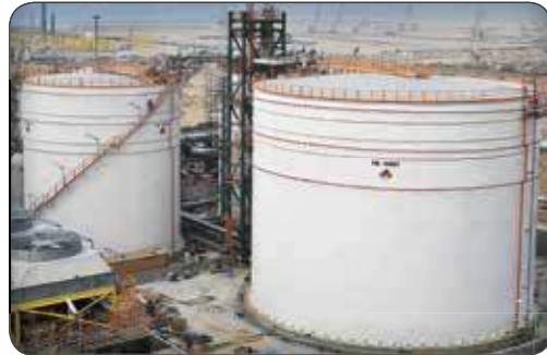
Storage Tank Marjan Petrochemical Co.
