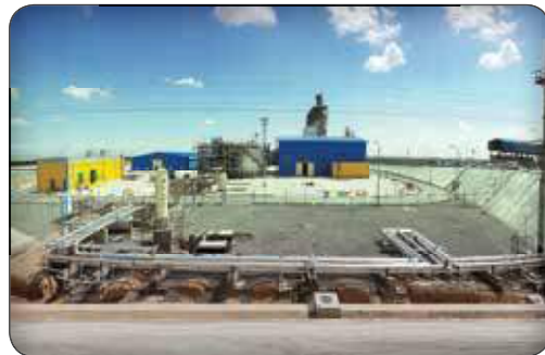
Installation of Sulfur Solidification Unit (SSU) Of Gasoil Refinery Project of Isfahan Refinery Company
