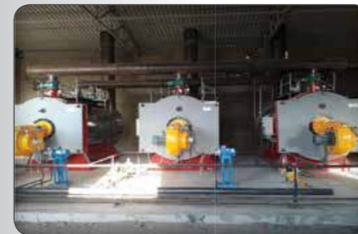
Gas-oil burner Type: MFGL800 Capacity: 6000000 kcal/h On pot abbant Project location: Shahrood Company: miami cheese
