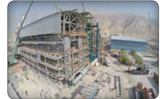
Reformer Marjan methanol plant
