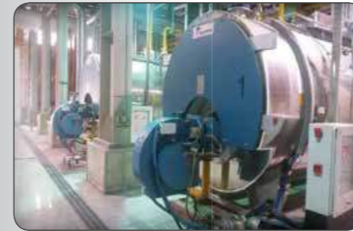
Gas-oil burner Type: MF GL 500 Capacity: 3500000 kcal/h Coroz company
