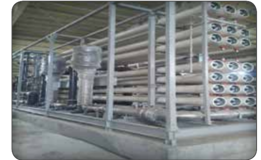
Water Treatment (Ro, Thermal Desalination, ...) Esfahan Refinery
