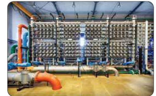
Water Treatment Package
