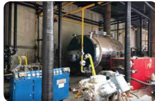
Thermal Oil Heater Fooman Shimi Main Factory
