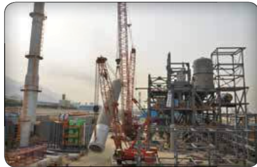
Installation of Urea Unit of the 3rd Phase of The Pardis Petrochemical Company (Capacity One Million Tons Per Year)
