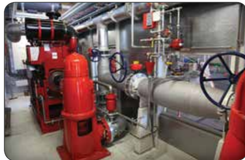
Fire Fighting Container Package for MAPNA Combined Power Plants
