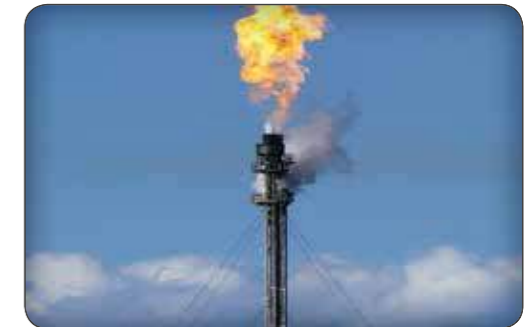
Flare Bid Boland Refinery
