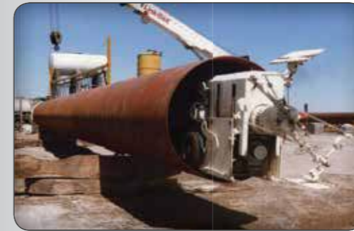
Cement Lining Plant Tehran-1995
