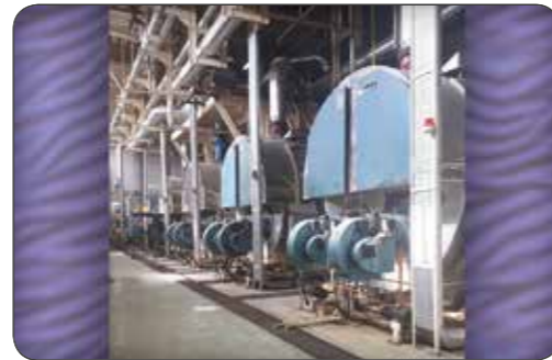
Three Pass Hot Water Boiler Irankhodro Factory (Khorasan)
