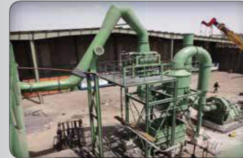
Dedusting System Mobarakeh Steel Co. (Kharazi Project)
