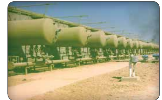
Gas Storage Plant Tehran-1984
