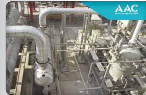
Water refrigeration package Different places
