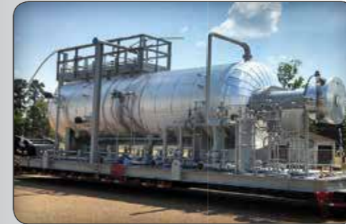
Oil Desalting Package
