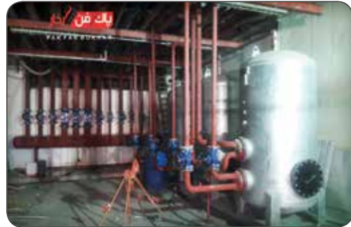
Three pass wet back steam boiler
