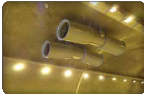
Tunnel ventilation, firefighting and automation
