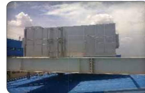
Air Handling Unit & Heat exchanger Saipa Citroen Co.
