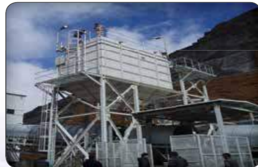
Bag Houses (Pulse & Reverse Air) Ardakan Pelletizing Plant Jovein, Abadeh, Delijan Cement Co., SUNGUN Copper Mine Industry
