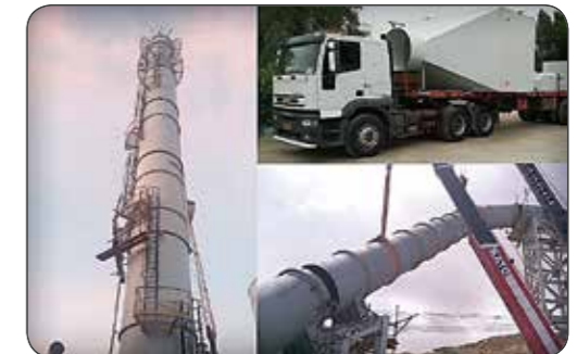
Stack & Duct – Sarcheshmeh Copper - NICICO
