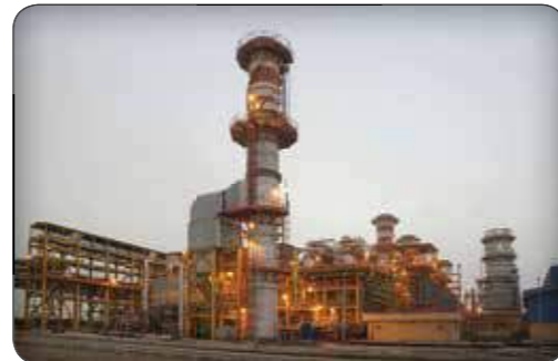
Package/Industrial Boilers Fajr 2 Petrochemical Project
