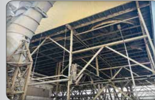
Turbine air intake cooling
