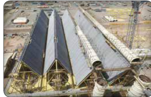
Air Cooled Condenser Parand
