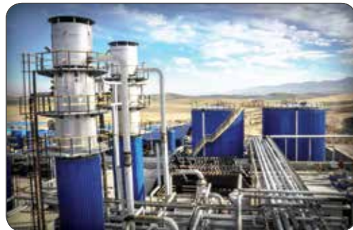
Bitumen Plant Soleymaniye-2012
