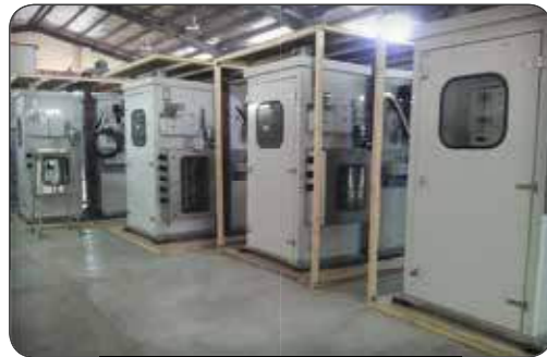
Continuous Emission Monitoring System/Flue Gas Monitoring System
