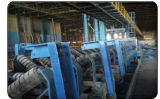
Manufacture of Conveying Systems & Hoppers over 1000 tons (Isfahan Zobahan Saba Steel Development Plan)
