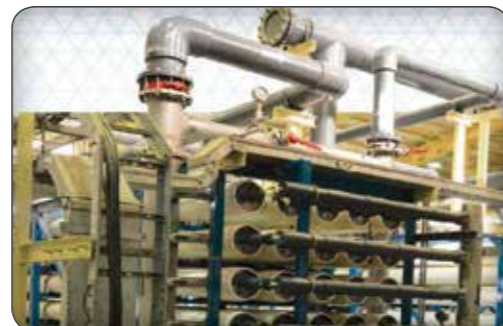
Sea Water Desalination System
