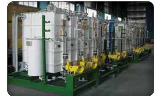
Chemical injection package Khesht oil field
