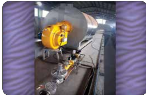
Gas burner Type: UDGL600 Capacity: 4000000 kcal/h On panel furnace Project name: Sepehr Varz Project location: Ahar
