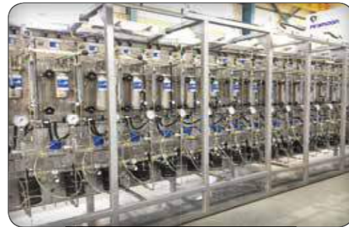
Sampling System/Steam and Water Analysis System
