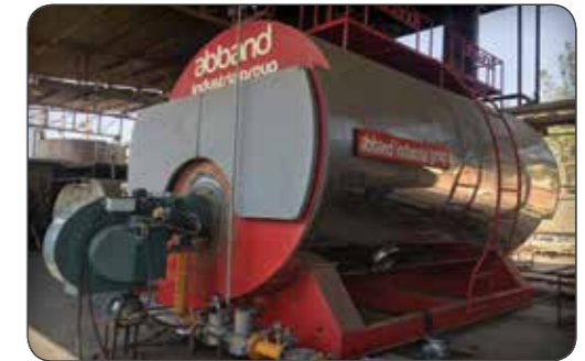
Gas-oil burner Type: MFGL800 Capacity: 6000000 kcal/h On pot abbant Project location: Shahrood Company: miami cheese
