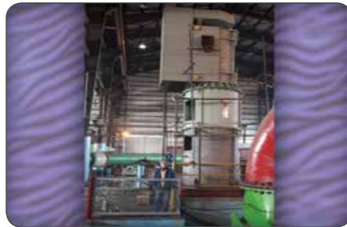
PERSIAN GULF STAR Refinery: Pump Model : VSP1-1200.1300 Capacity: 12200 m 3 /h, Head: 54 m, Power: 2.5 MW
