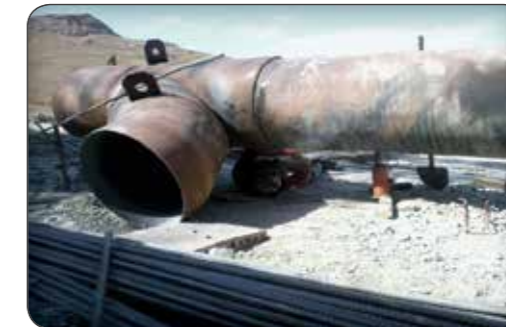
Hydromechanical and electrical equipment of Siyazakh Dam
