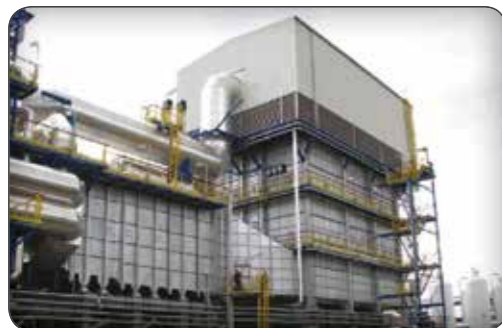
Waste Heat Boilers
