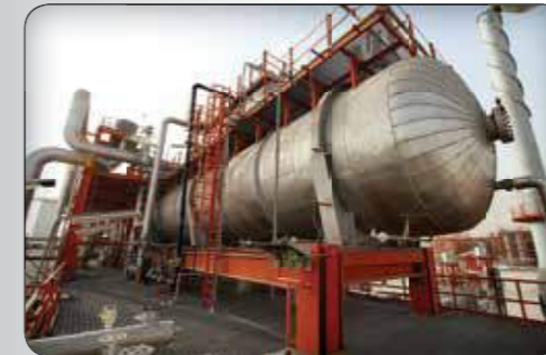
De-aerator Phase 15&16 South Pars plant
