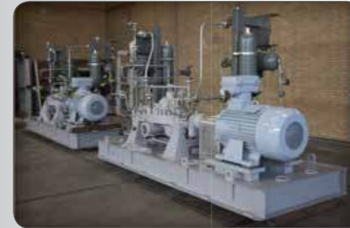
BB3 Pumps for Bouali Sina petrochemical Project
