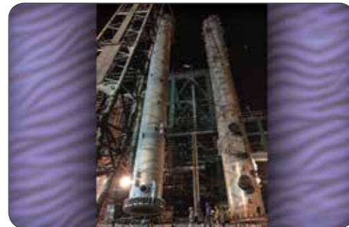
Marjan Petrochemical Company Vertical Shell & Tube Heat Exchanger
