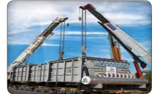
Furnace / combustion systems / Incinerator package / reformers (Marjan Methanol Plant)
