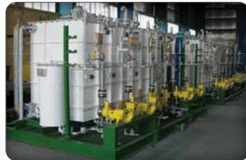
Chemical Injection Package
