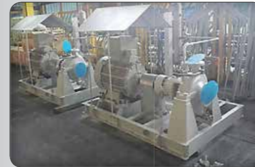
ENTEKHAB Petrochemical Project Pump Model: CP-80.315 Capacity: 132 m 3 /h, Head: 139 m, Power: 90 Kw
