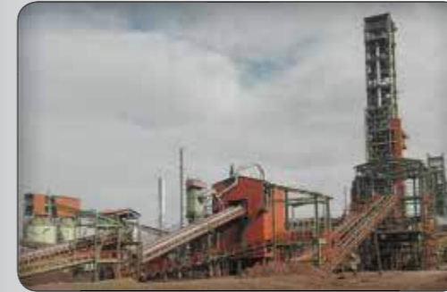
Material Handling System GISD Mega Module Kowsar- Sirjan
