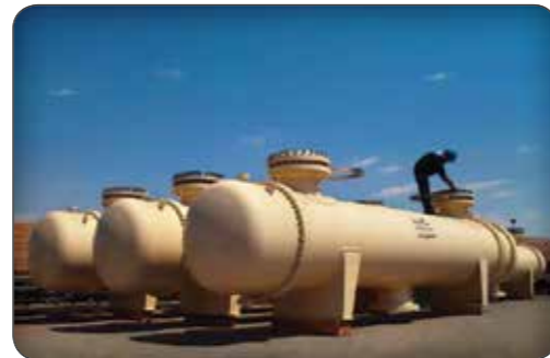
Shell and Tube Heat Exchanger Boushehr
