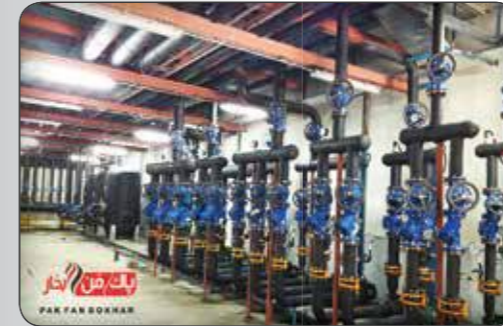
Oil heater boiler
