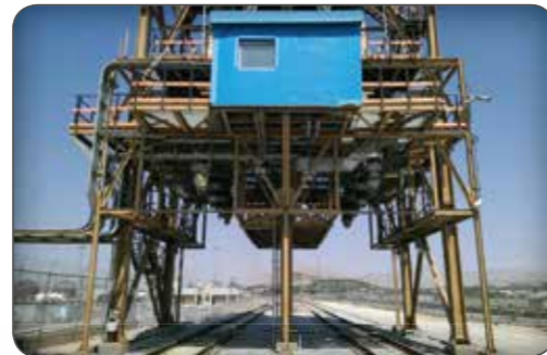
Wagon Loading Stations
