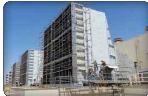
Construction of Evaporative Cooling Systems for 160MW Gas Turbines Inlet Air (Ifa Sanaat Taba Company).
