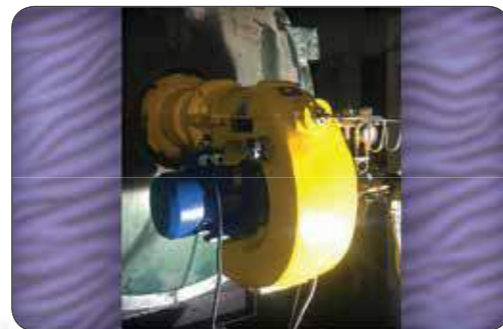
Gas-oil burner Type: UDGL250-1 Capacity: 1800000 kcal/h On horizontal hot oil furnace Project location: Booshehr Petro rama company
