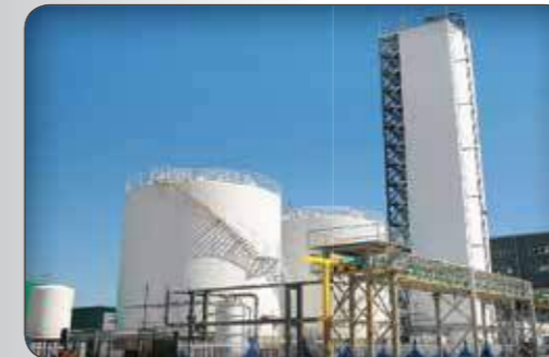
Air Separation Unit Bandar Abbas Gas Condensate Refinery
