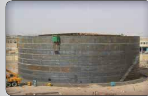
Construction of 2820m3 Floating Roof Tanks- Zabol, Mahshahr, Kish, Bandar Lengeh & Qeshm
