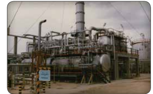
Sulfur Recovery Plant Arak-1992
