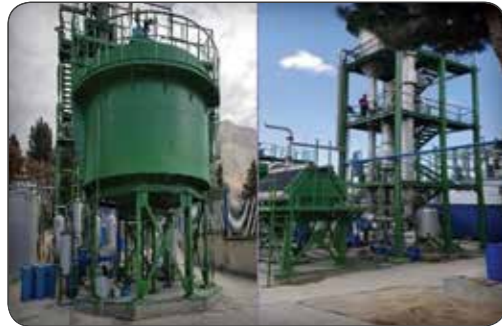
Water Treatment plant (Zero Liquid Discharge)
