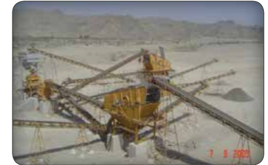
Customer Kosar jahan Co. in Chababar Installations and materials manufacturing machinery
