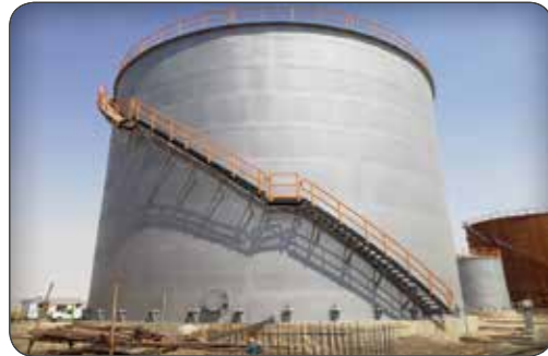
Storage Tank – NGL3200 - PEDEC
