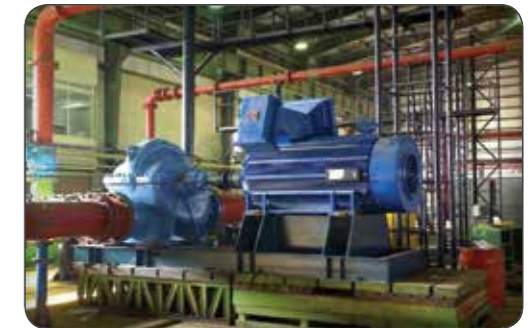
ILAM Petrochemical Project Pump Model: VENUS 1-500.800 Capacity: 4200 m 3 /h, Head: 50m, Power: 850 kw
