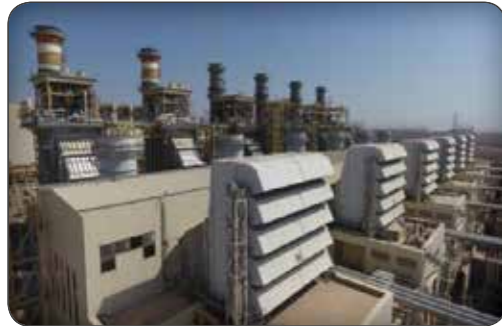
Equipment of Thermal Power Plants
