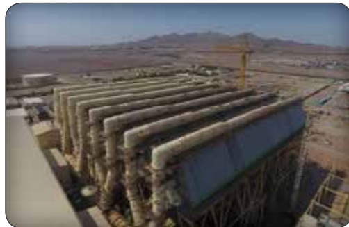
ACC-Dry Cooling Systems Parand Combined Cycle Power Plant
