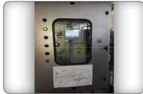
Waste Water Analyzers (TO, BOD, COD, TSS, ...)
