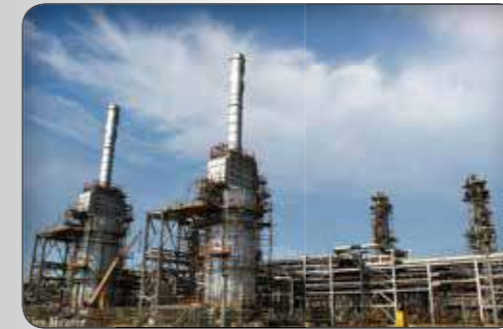
Fire Heater Reboiler Heater
