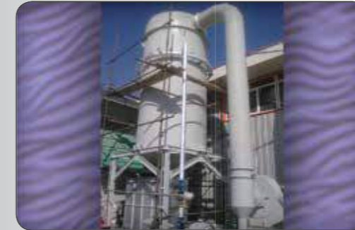
Packed Towers Ettehad Lent Pishro Sanat Co.
