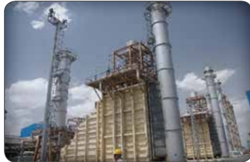
Heat Recovery Steam Generator(HRSG/ WHB) Montzer Ghaem Power plant
