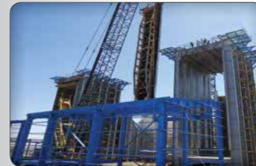
Fabrication and Installation of Steel Structure and Equipment of Several Power Plant in Iran
