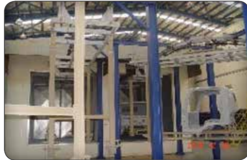
Complete Paint Shop (PT&ED) Bahman Diesel PT & ED Line
