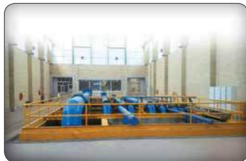
Hydraulic test kind of pump and electro pump
