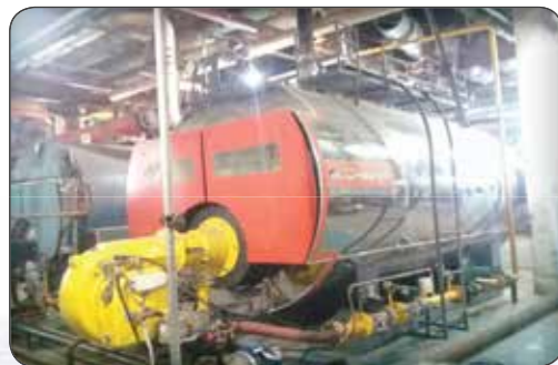
Gas-oil burner Type: UDGL600 Capacity: 4000000 kcal/h On pot Dabo Sanat Project location: mehr abad airport
