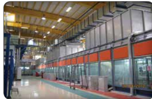
Bumper Painting Plant SAIPA-2008
