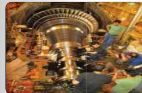
Overhaul, Repair and Maintenance of various types of Gas turbines and Steam turbines. Avon 1535 (NISOC) Shinko (NITC) MGT30- DU80 (NIGC & PARSIAN Refinery)
