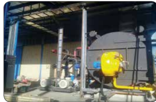
Gas-oil burner On hot oil furnace Type: UDGL600 Capacity: 4000000 kcal/h Project name: wood and chip point Project location: Semnan
