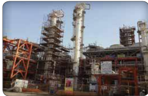
Completion of Work, Pre-Commissioning & Punch List Removing and Start Up Units No 107,116,183 Of Phase 13 Of South Pars Refinery
