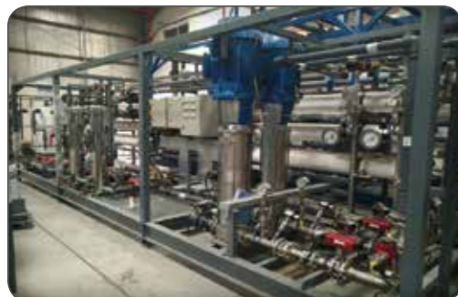
Water Treatment Package West Karoon WTP Project
