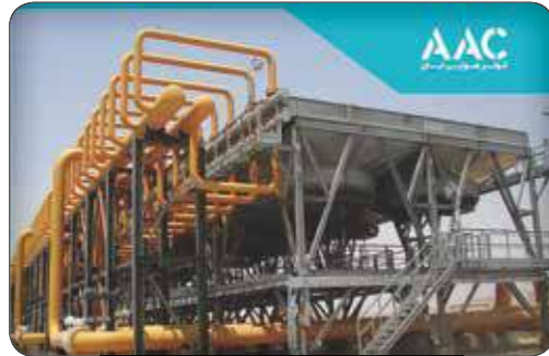
Air Cooled Heat Exchanger ODCC
