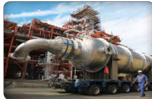
Process Reactor (Bushehr Methanol Plant)
