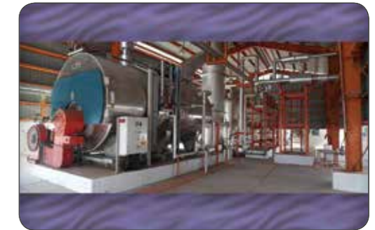
Condensate Tank, Boiler & Other Boiler Room Accessories Rosemond Petrochemical Of Bushehr
