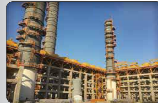
Construction of AG Piping, Civil, Steel Structure, Equipment of Apadana Petrochemical Co.
