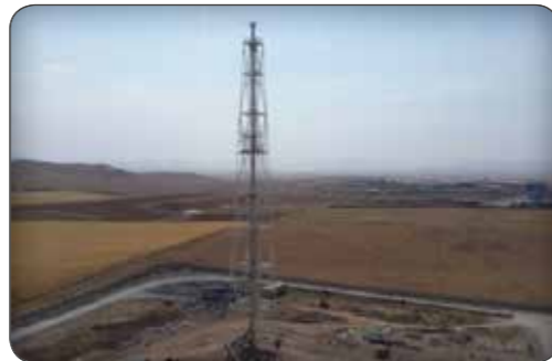
Flare Stacks & Incinerators (Manufacturing of Flare Stack for Di- Polymer Arya Petrochemical Plant)
