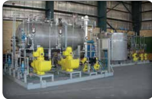
Chemical Injection Package
