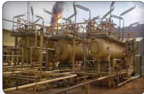
Oily Water Treatment Package
