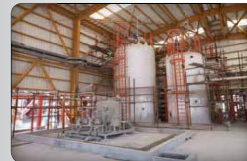
De-Oiling Phase 15&16 South Pars plant
