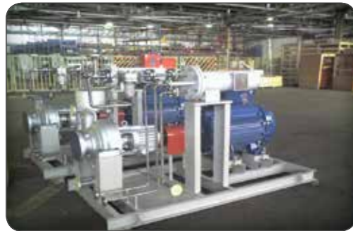
SHAZAND Refinery Pump Model: CP-200.565 Capacity: 320 m 3 /h, Head :88m , Power :90 kw
