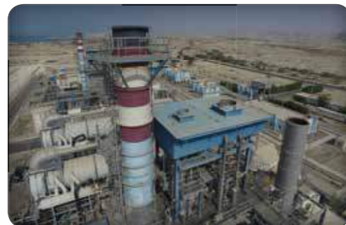
CHP Boilers Qeshm power and water plant
