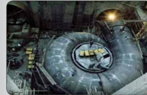
Hydraulic Power Plant and Equipment Turbine Karoun 3 Dam
