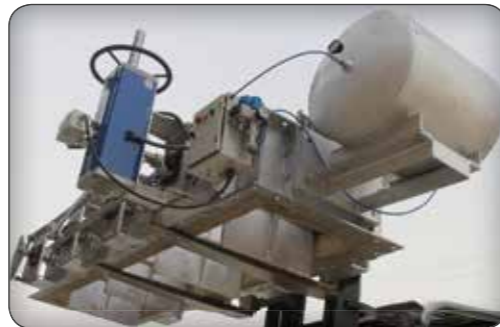
Damper valve, Louvers and silencer
